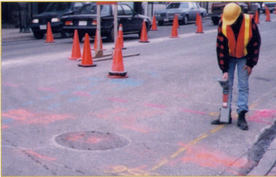
FIGURE 2 Locating multiple underground facilities as part of a pre-engineering design utility mapping investigation.
