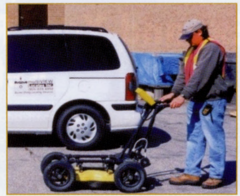
FIGURE 3 Acquiring ground penetrating radar data over a series of parallel survey lines to map the underground infrastructure.
